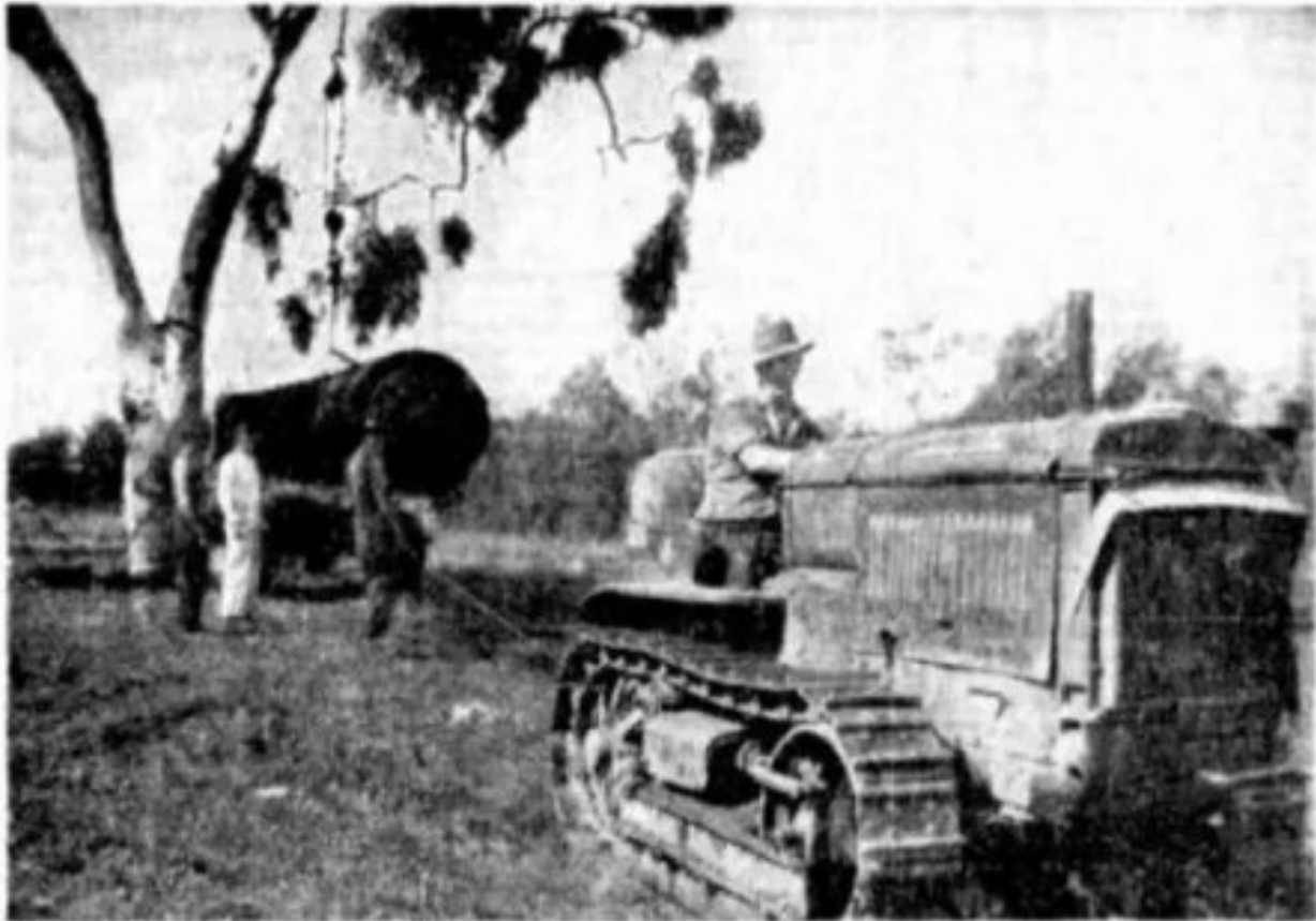
NEW BOILER FOR COMET PUMPING PLANT.—The Railway Department removing the old locomotive boiler from the pumping station on the weir in the Comet River. Here is the old boiler suspended from the branch of a tree preparatory to being loaded on a timber jinker. The new boiler was placed into position last week.
